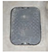
Floor plate cover for backwater valve.
